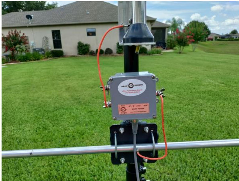
Figure 2: My vertical dipole antenna current configuration.
